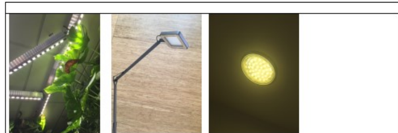
Use of LED lighting in offices
